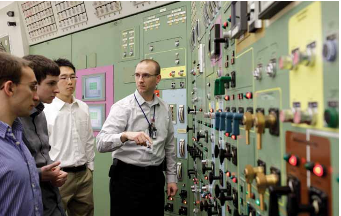
Michael Gillin '99 COE, '04 MBA, senior manager of Plant Engineering at Exelon’s Limerick Generating Station, gives students a tour of the simulator building.
